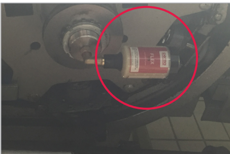
Drive pulley bearing lubrication on an oven
